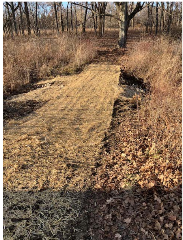
Initial culvert and stone installation and finish grade with topsoil, seed, and straw cover at LeRoy Oakes FP.
